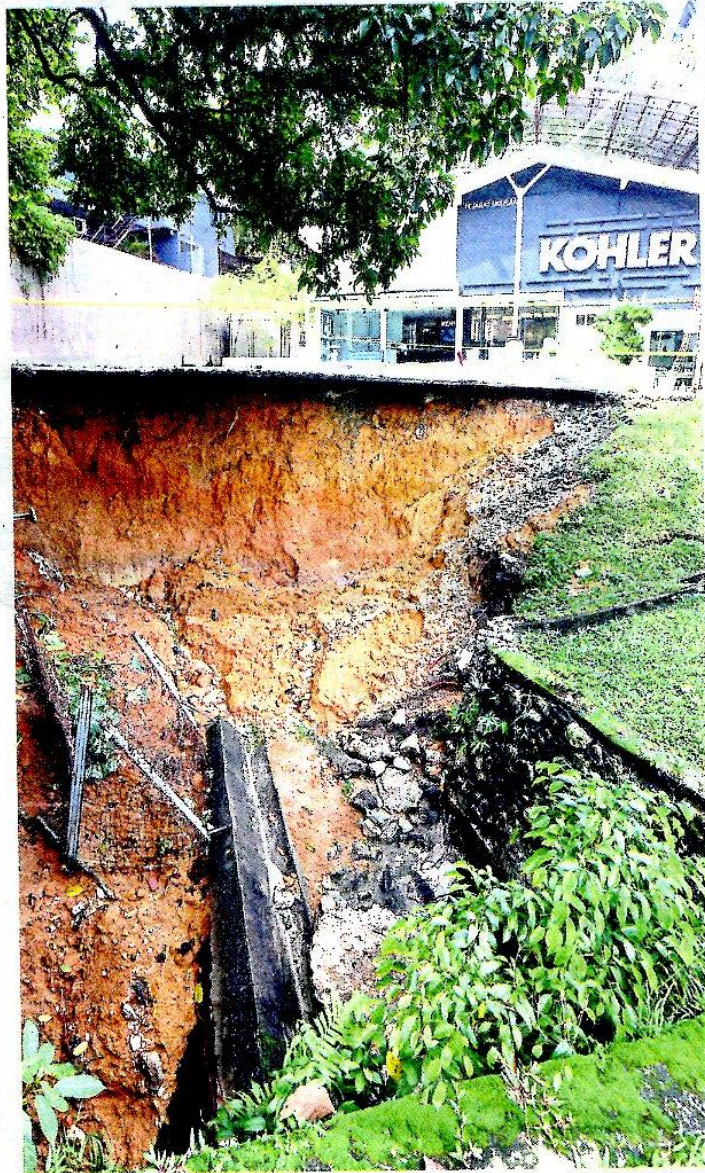
The landslip happened outside the showroom in Section 16, Petaling Jaya.
